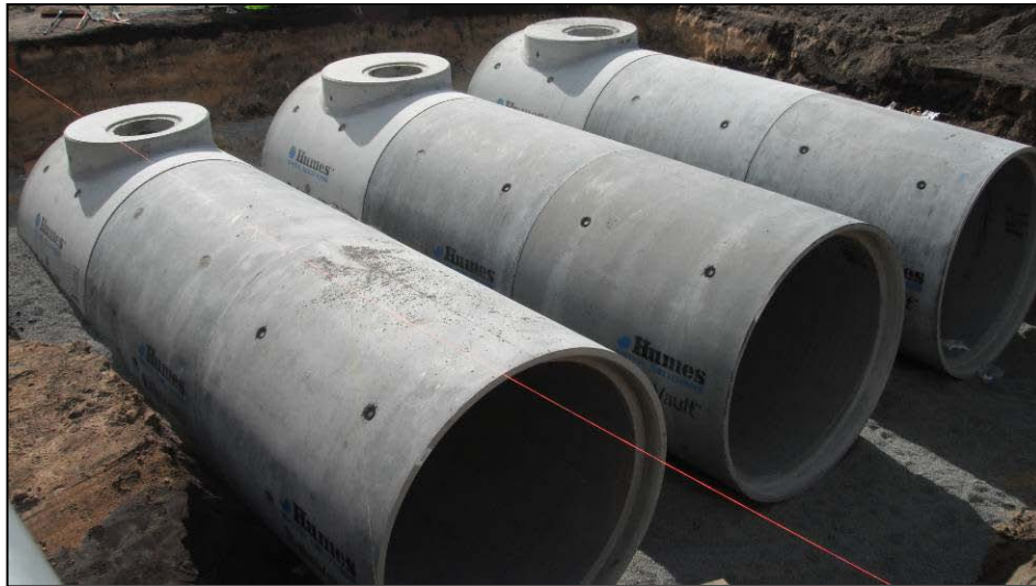
Photo of new storm water storage tank system
