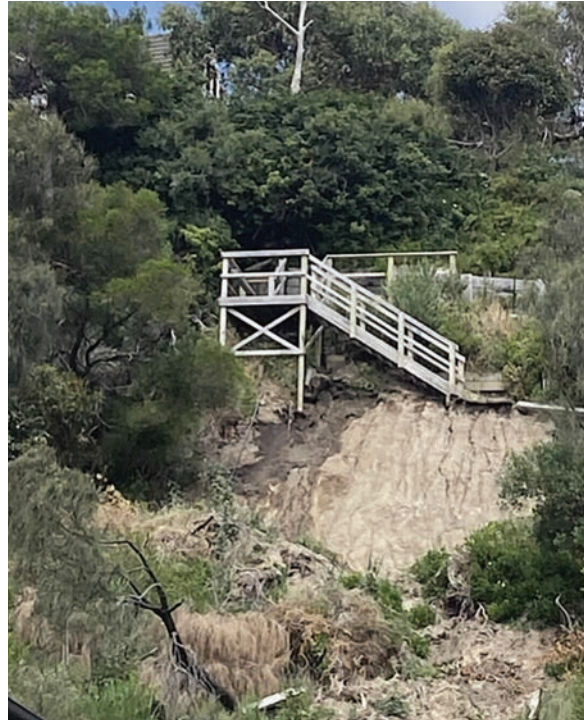
FIGURE 3.22: WET PATCH UNDER STAIRCASE ON 10–12 VIEW POINT ROAD. 252
