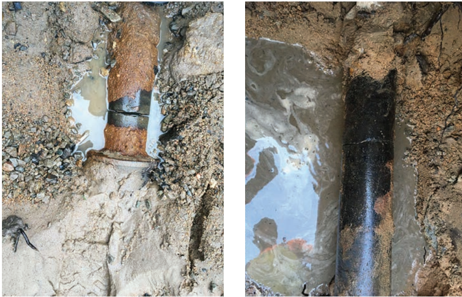
FIGURE 3.14: IMAGES OF THE BREAKS ALONG THE PIPE. 125
