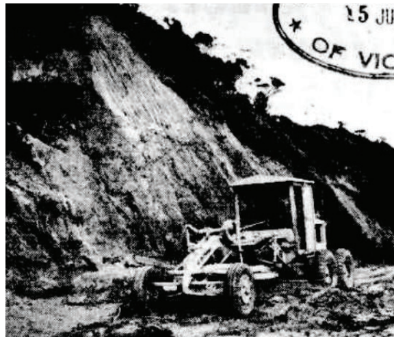
FIGURE 3.3: CLEAN-UP OF A CUTTING FAILURE ON POINT NEPEAN ROAD NEAR ANTHONY'S NOSE. 7
