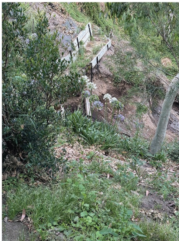
FIGURE 3.41: PHOTOGRAPH TAKEN BY MR BORGHESI OF THE RETAINING WALL FAILING ON 12 JANUARY 2025. 705
