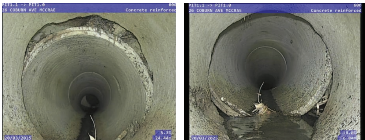
FIGURE 4.23: BREACHES IN THE STORMWATER PIPE LOCATED AT BROWNE STREET. 180
