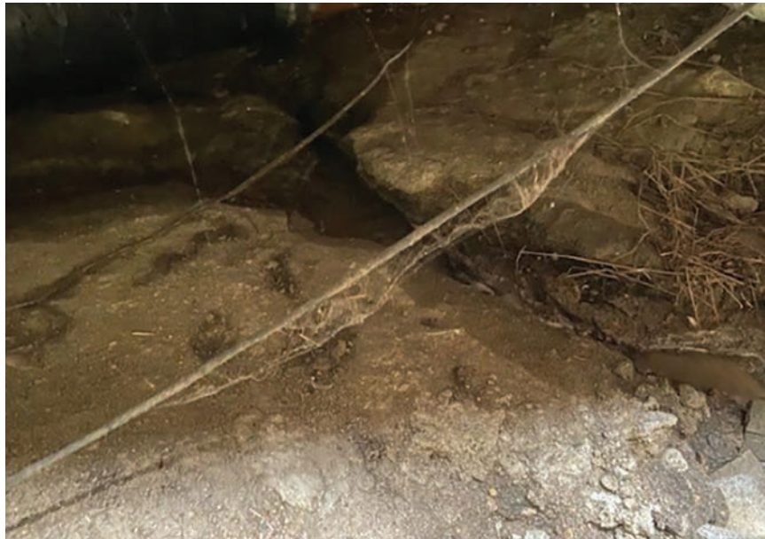
FIGURE 3.35: PHOTOGRAPH OF SCOUR LINES UNDERNEATH 3 PENNY LANE. 557
