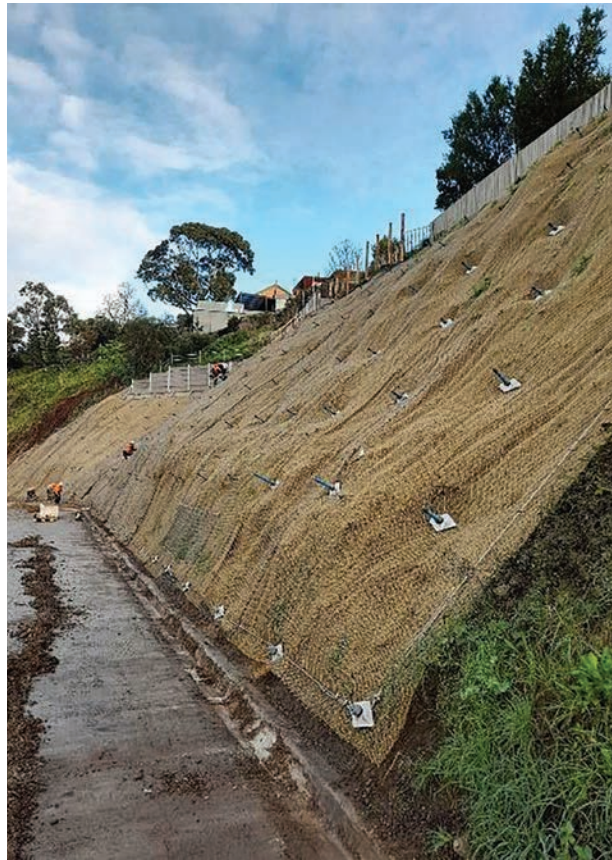
FIGURE 5.8: COMPLETED SLOPE MITIGATION WORKS ALONG THE HAMILTON HIGHWAY USING SOIL NAILS AND MESH. 75
