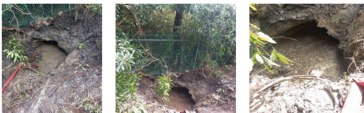
FIGURE 3.31: PHOTOGRAPHS OF BURST WATER MAIN SITE ON 31 DECEMBER 2024. 470
