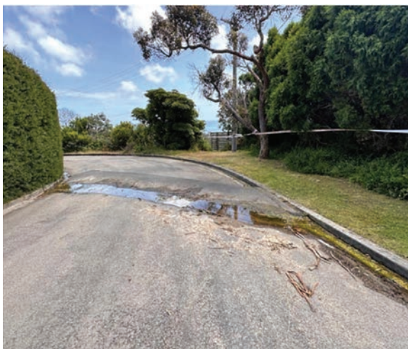
FIGURE 3.19: WATER RUNNING ALONG THE KERB ON VIEW POINT ROAD. 215
