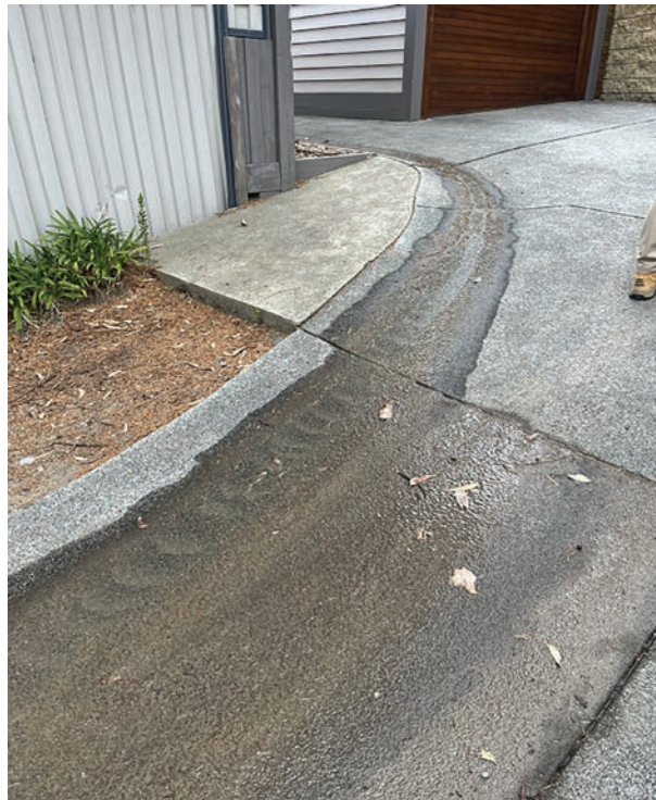
FIGURE 3.38: PHOTOGRAPH TAKEN BY MR ROTTER OF THE WATER FLOWING FROM THE DRIVEWAY OF 3 PENNY LANE DOWN PENNY LANE ON 9 JANUARY 2025. 635
