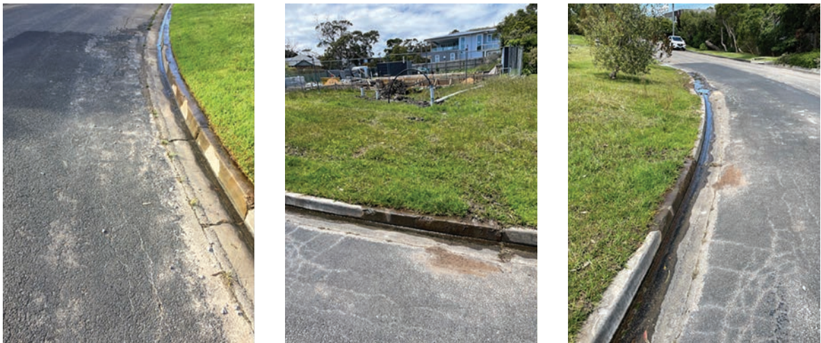
FIGURE 3.11: PHOTOS OF THE KERBS DURING THE DEVELOPMENT OF 7 PROSPECT HILL ROAD BETWEEN 5 MAY 2021 AND 11 NOVEMBER 2021. 107
