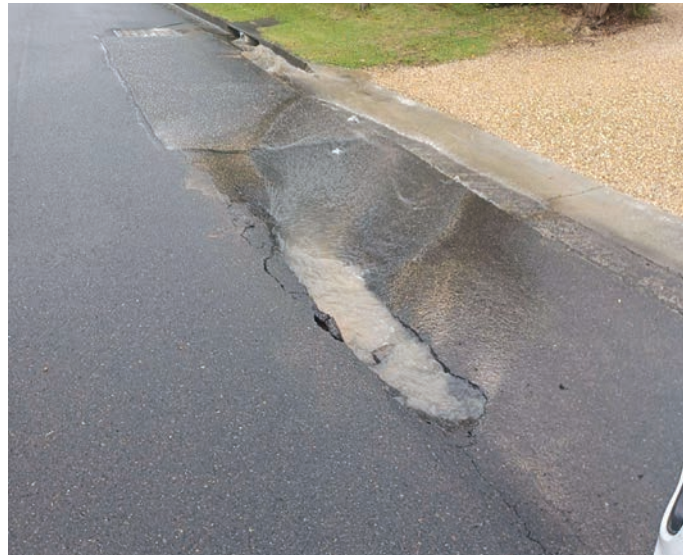
FIGURE 3.12: PHOTO OF DEFECT IN TARMAC AND WATER FLOW ON COBURN AVENUE. 117
