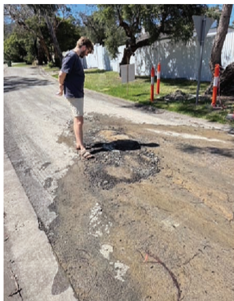
FIGURE 3.29: WATER SURFACING OUTSIDE 3 CHARLESWORTH STREET. 385
