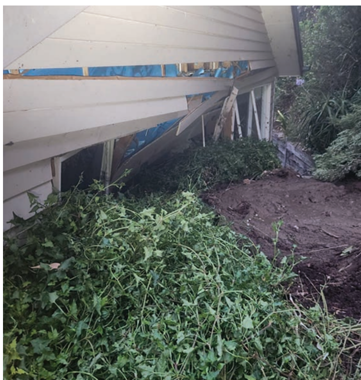
FIGURE 3.34: PHOTOGRAPH OF THE REAR OF 3 PENNY LANE FOLLOWING THE 5 JANUARY 2025 LANDSLIDE. 548
