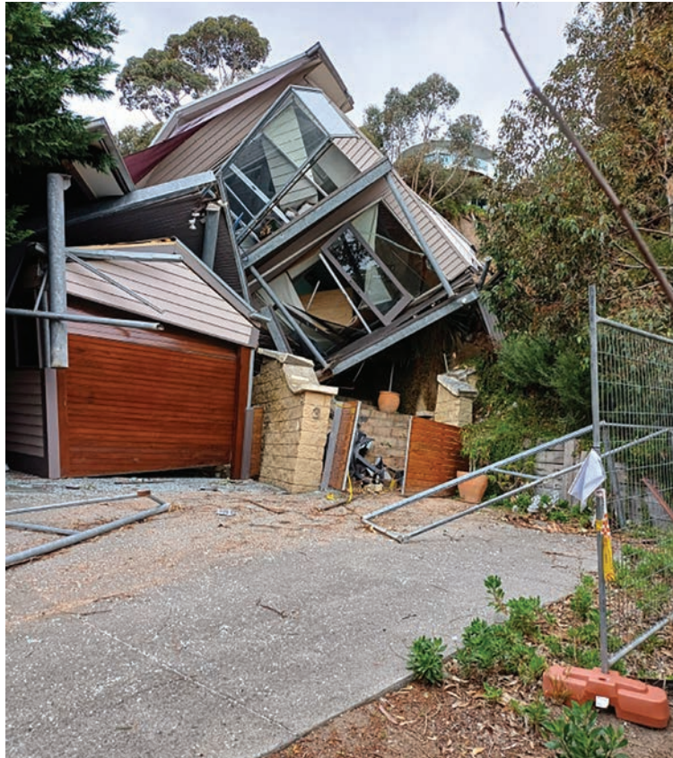
FIGURE 3.45: PHOTOGRAPH OF 3 PENNY LANE FOLLOWING LANDSLIDE ON 14 JANUARY 2025. 745
