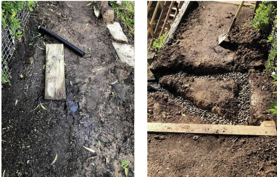
FIGURE 3.9: COMPARISON BETWEEN THE HILLSIDE PATH PRE AND POST INSTALLATION OF THE AGRICULTURAL DRAINS. 99
