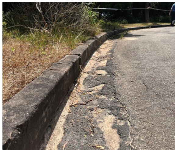
FIGURE 3.20: CRACKS AND PATCHING ALONG THE KERB OF VIEW POINT ROAD. 216
