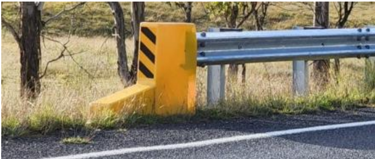
Figure 3-5 End Terminal on Road Barrier
