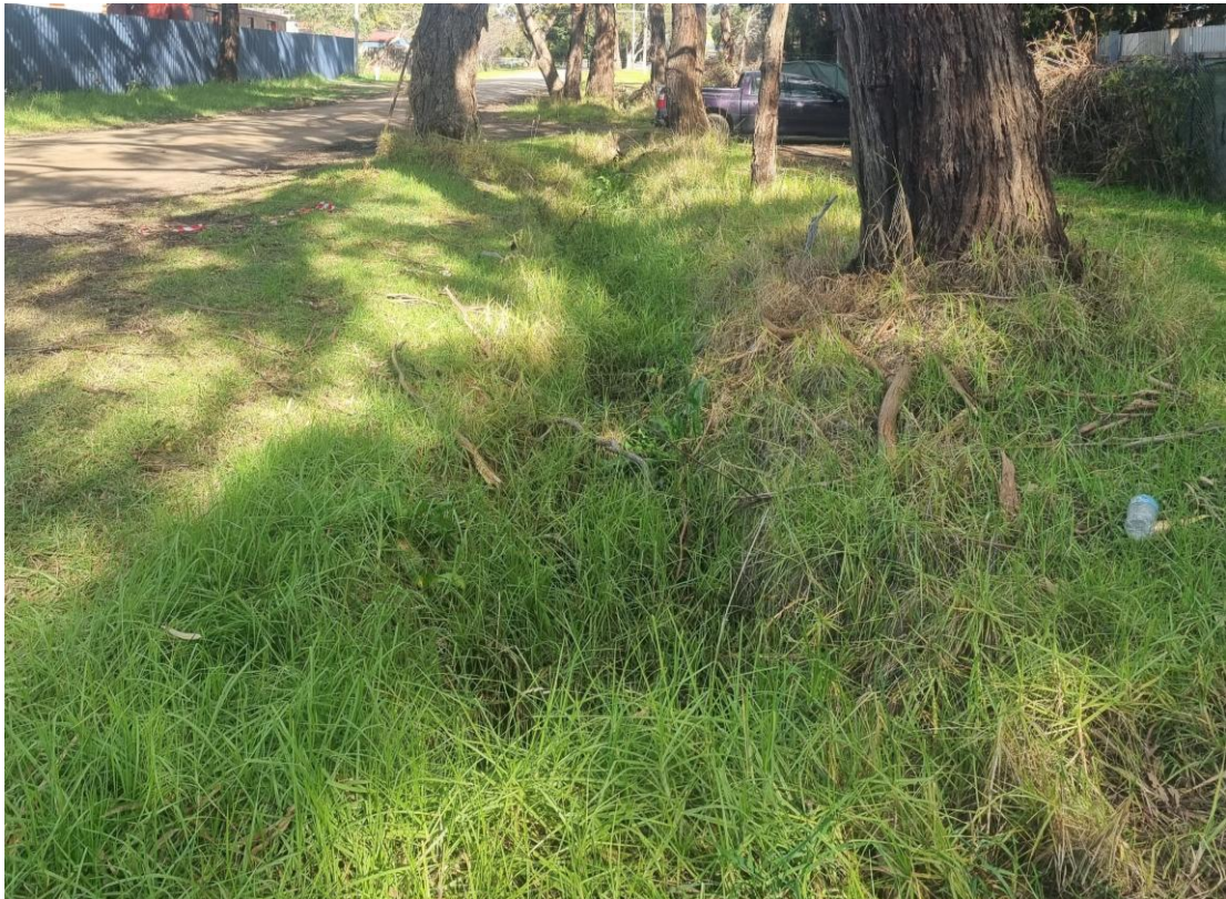
Figure 07 – Open channel drainage in the northern end of 6 Cooma Street.
