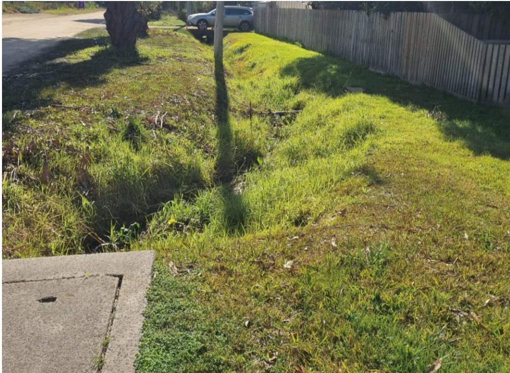
Figure 10 – Photo of existing open channel drainage within Glossop Street where it commences from the drainage pit at the Disney Street intersection.
