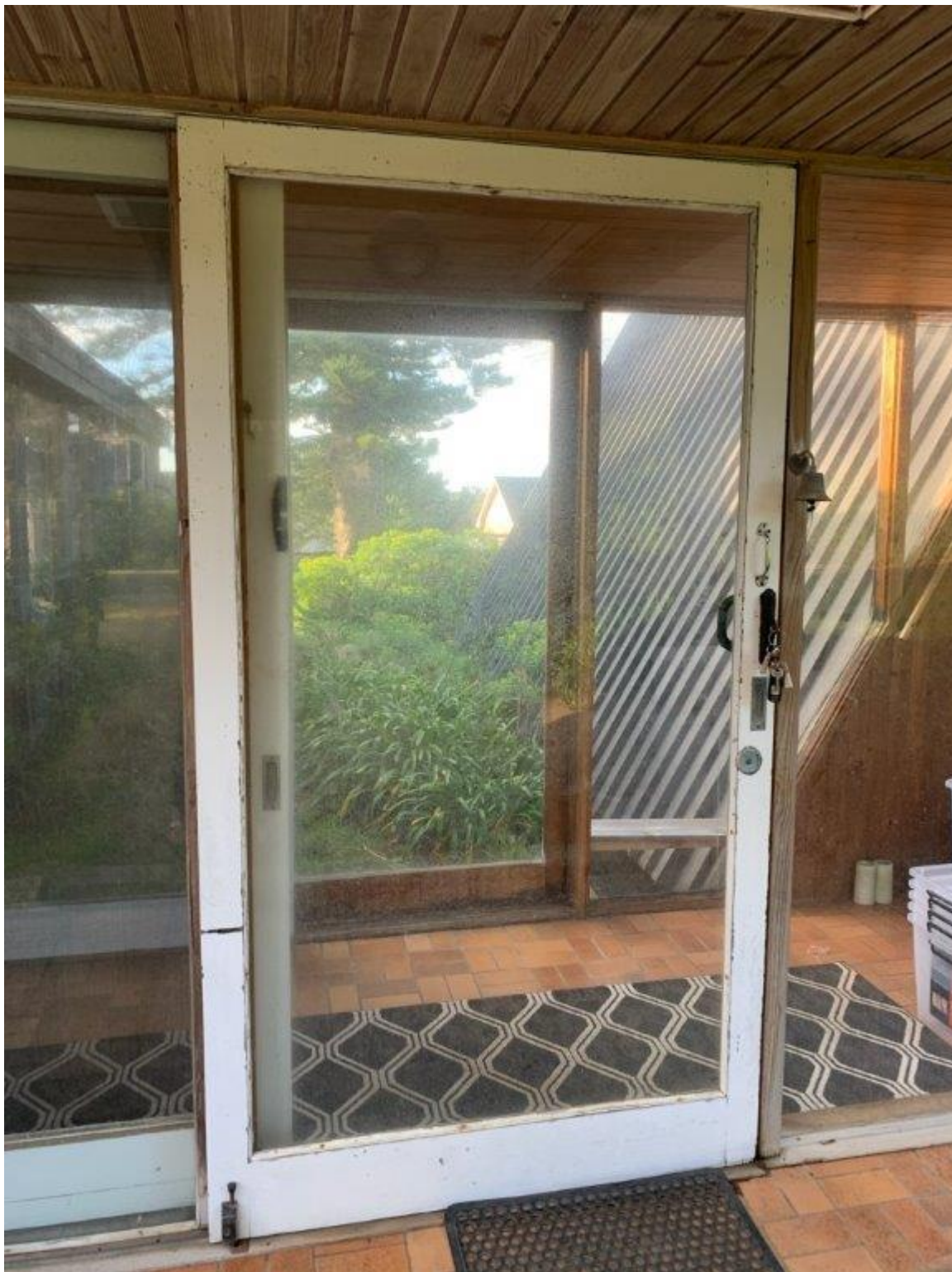
Front door; injury risk, often unable to close and lock, in need of constant repair
