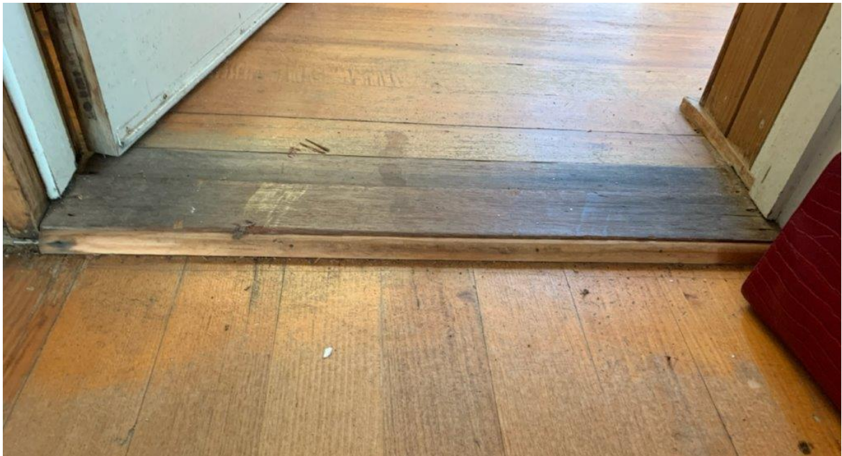
Living room doorway; trip hazard
