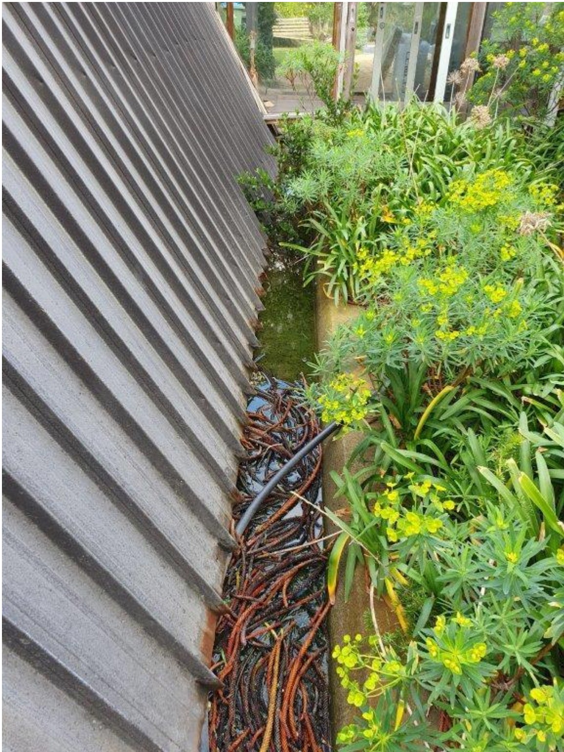
Aframe gutters; stagnant water, drainage not occurring
