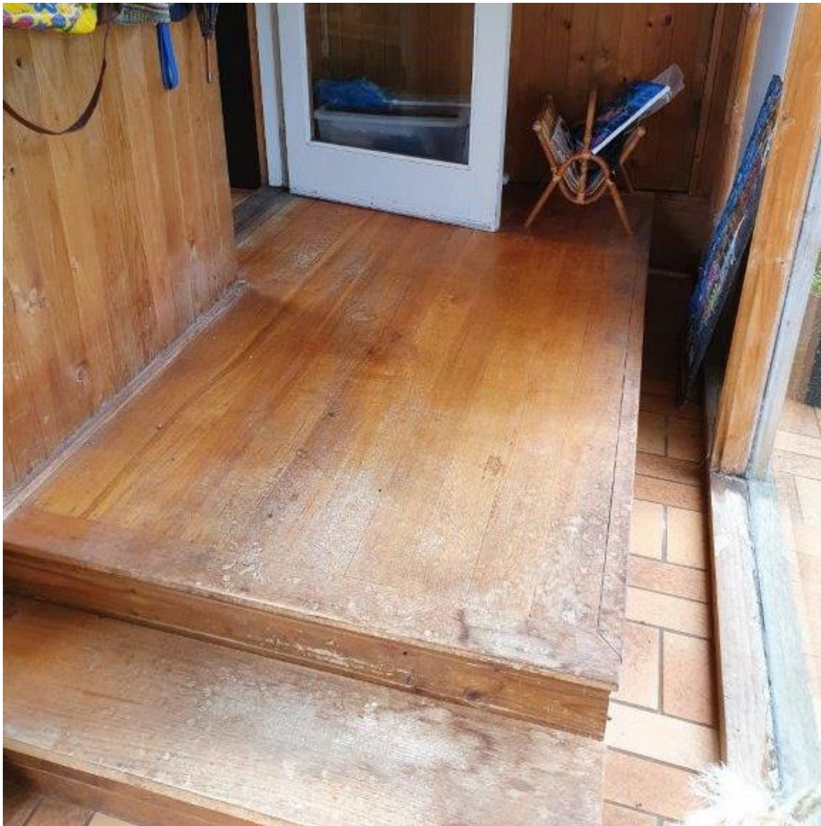
Passageway landing; water damage, fall and trip hazards
