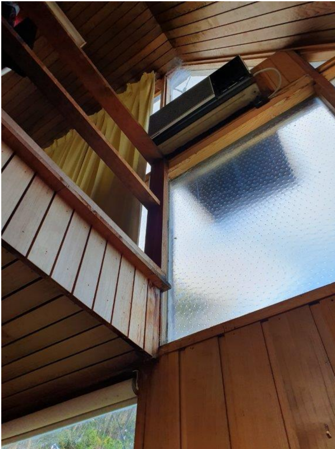
Aframe loft: water damage
