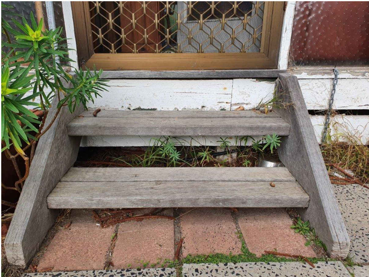
Aframe back steps; building movement, fall hazard, weather damage
