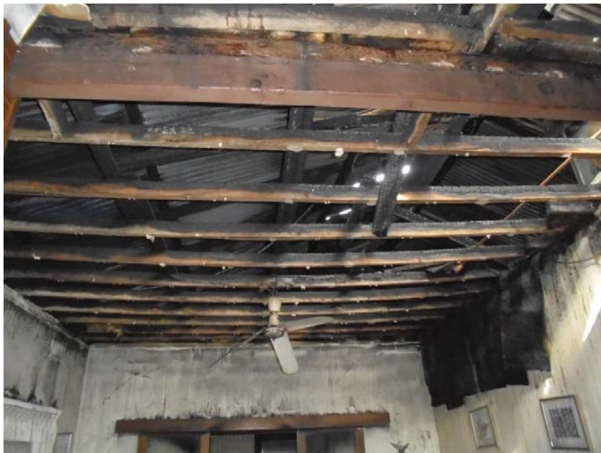
Significant damage to roof and walls of lounge room
