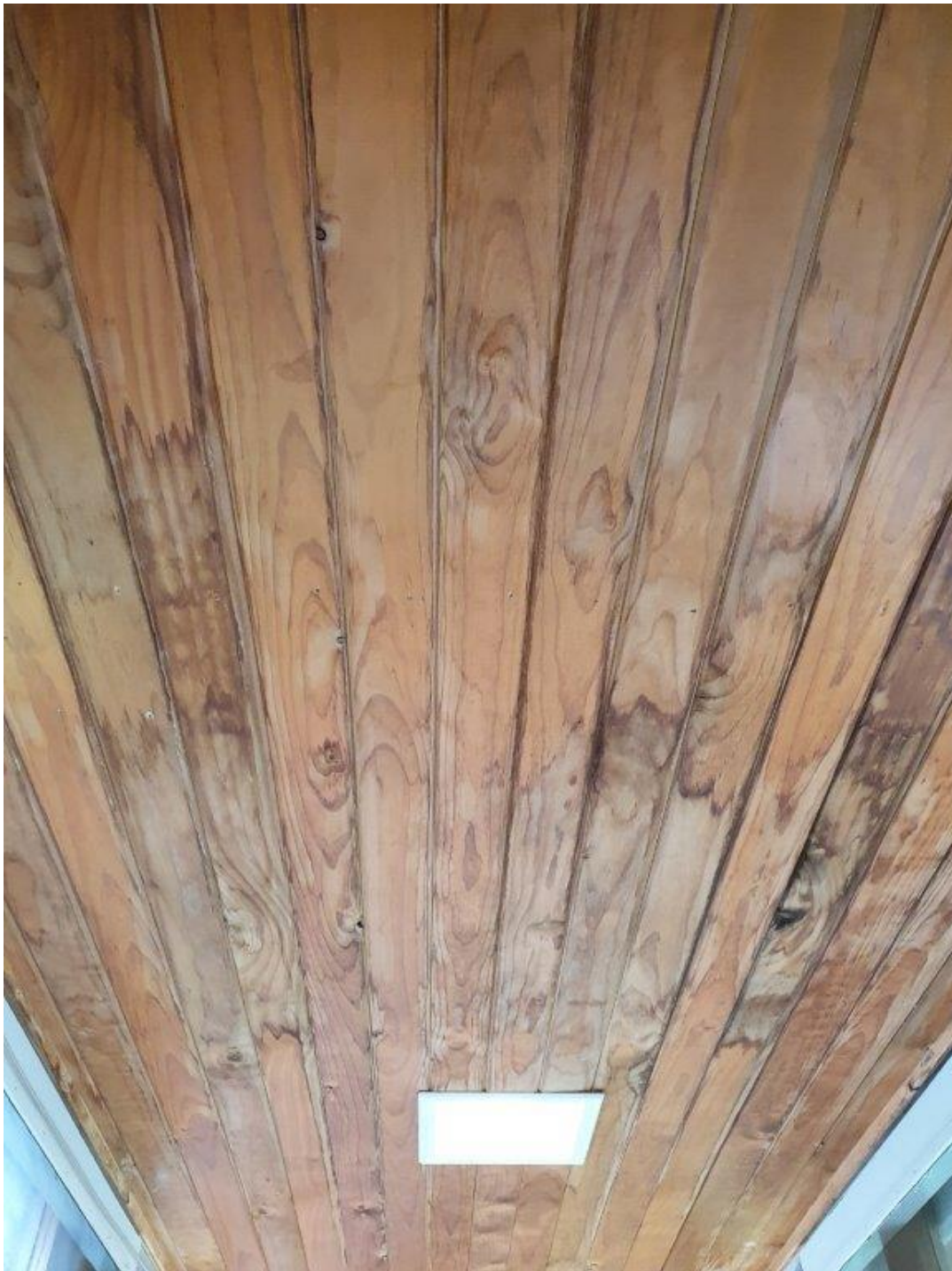
Passageway ceiling: water damage
