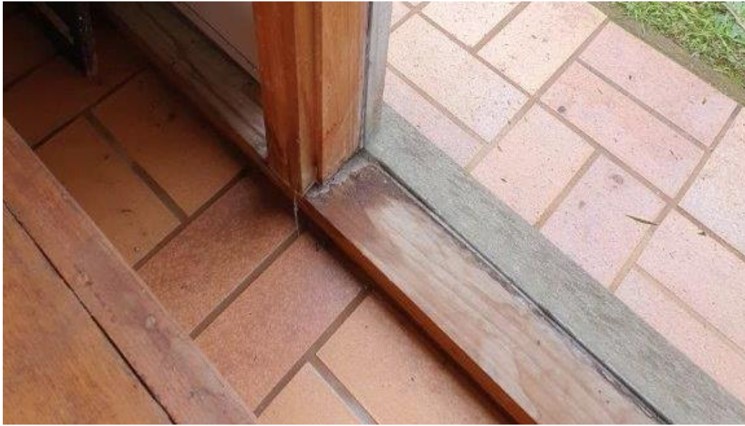
Passageway: water damage
