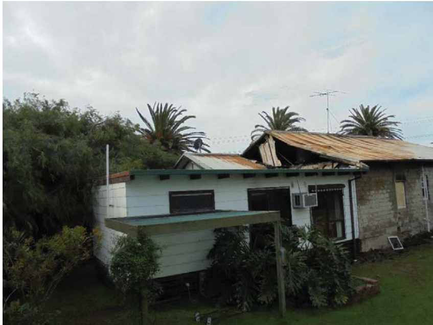
Damage to roof as can be seen from rear of building
