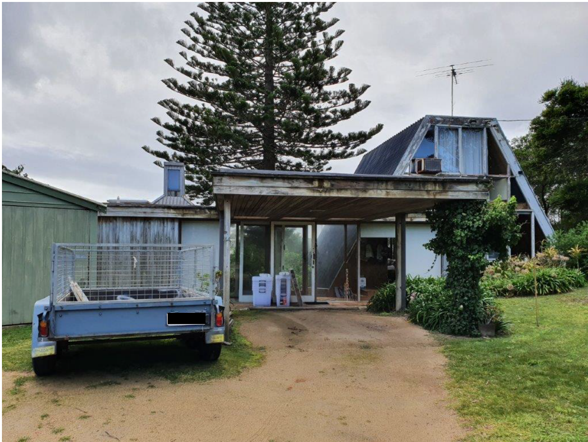
Front of property showing exterior weather damage
