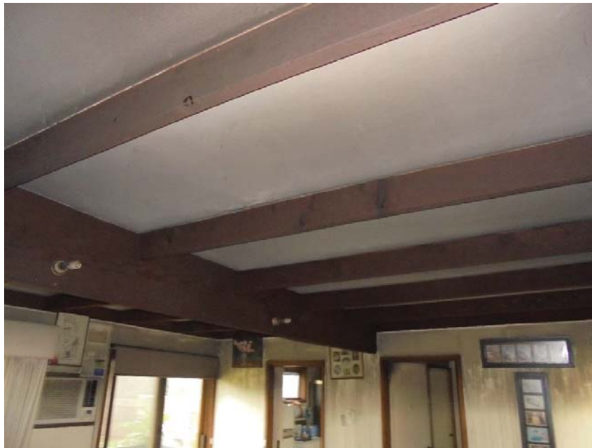
Soot damage to ceilings and walls
