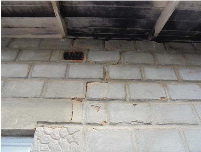
Cracking to block walls – pre-existing issue
