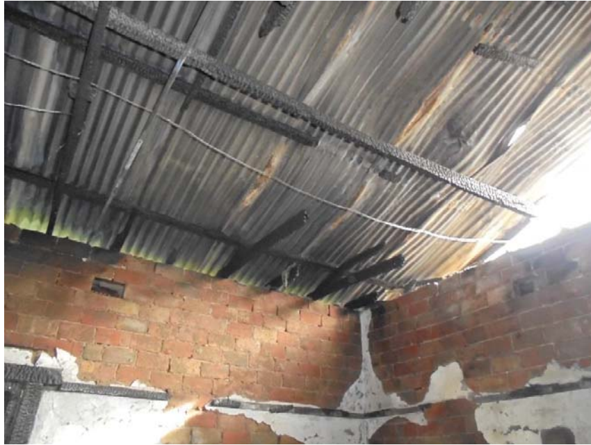
Unsupported roof sheeting
