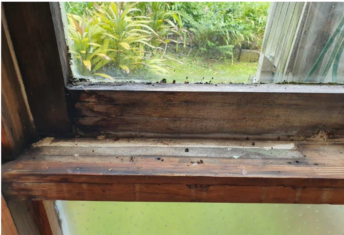
Aframe living room window: water damage
