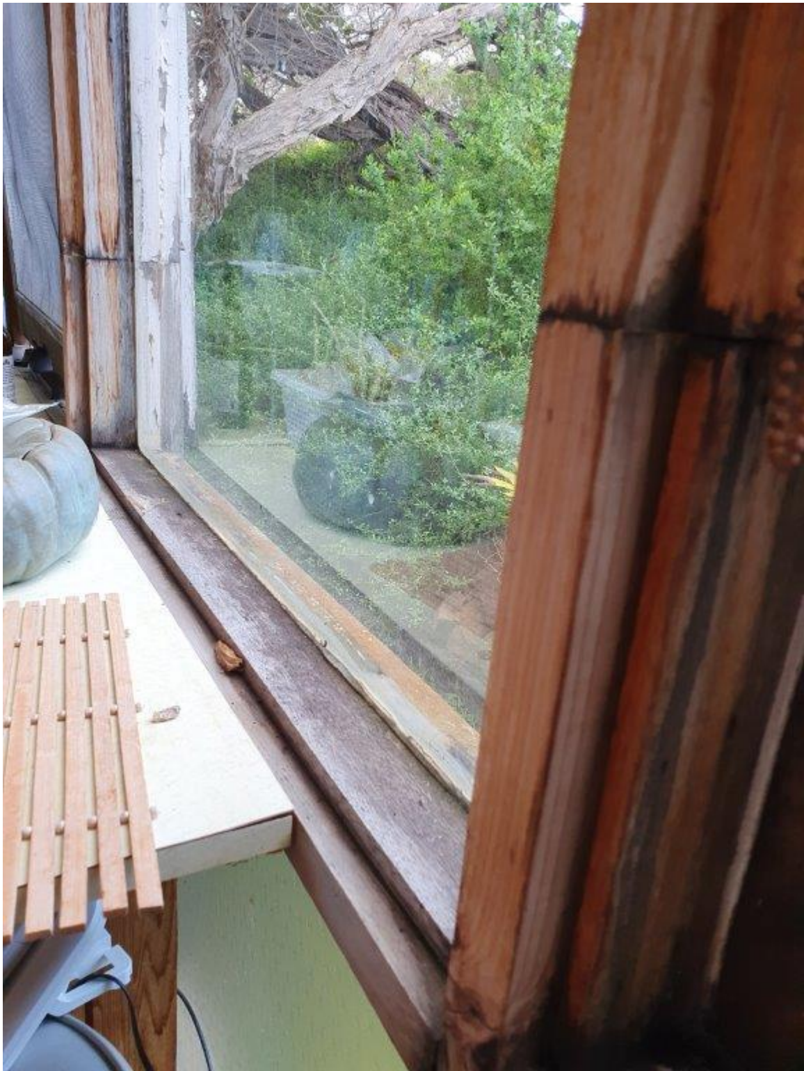
Aframe kitchen window: water damage
