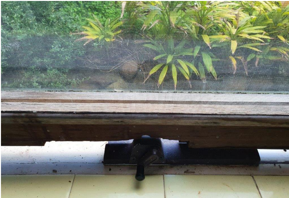
Aframe kitchen window: damage
