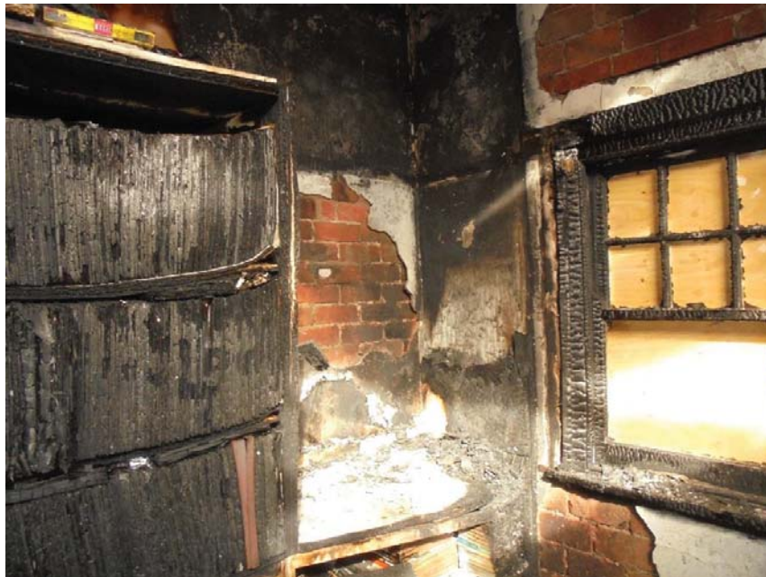
Location of fire ignition point
