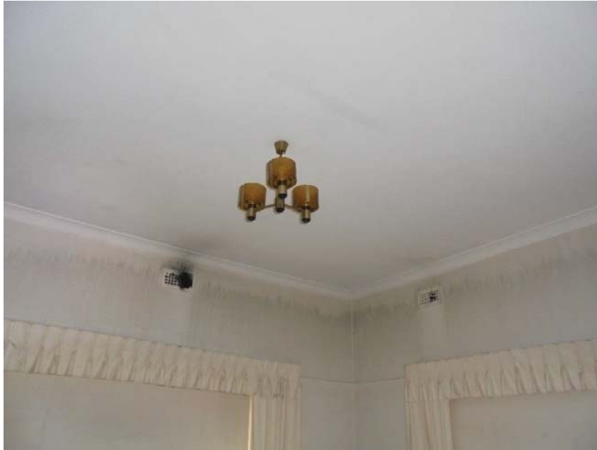
Soot and water staining to bedroom walls and ceiling
