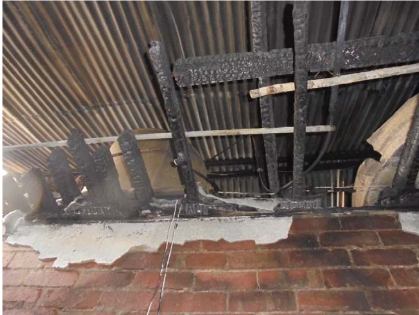
Significant damage to roof frame
