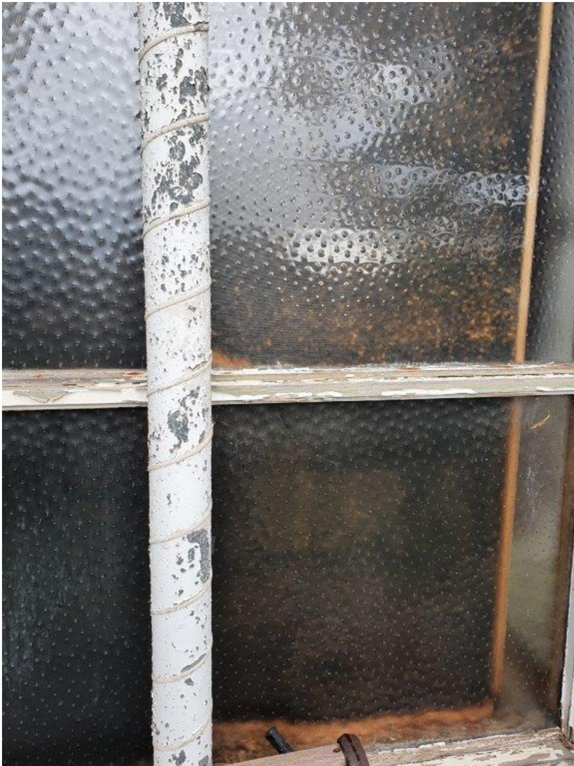
Aframe window outside second bathroom: mould, water damage, rust, weather damage
