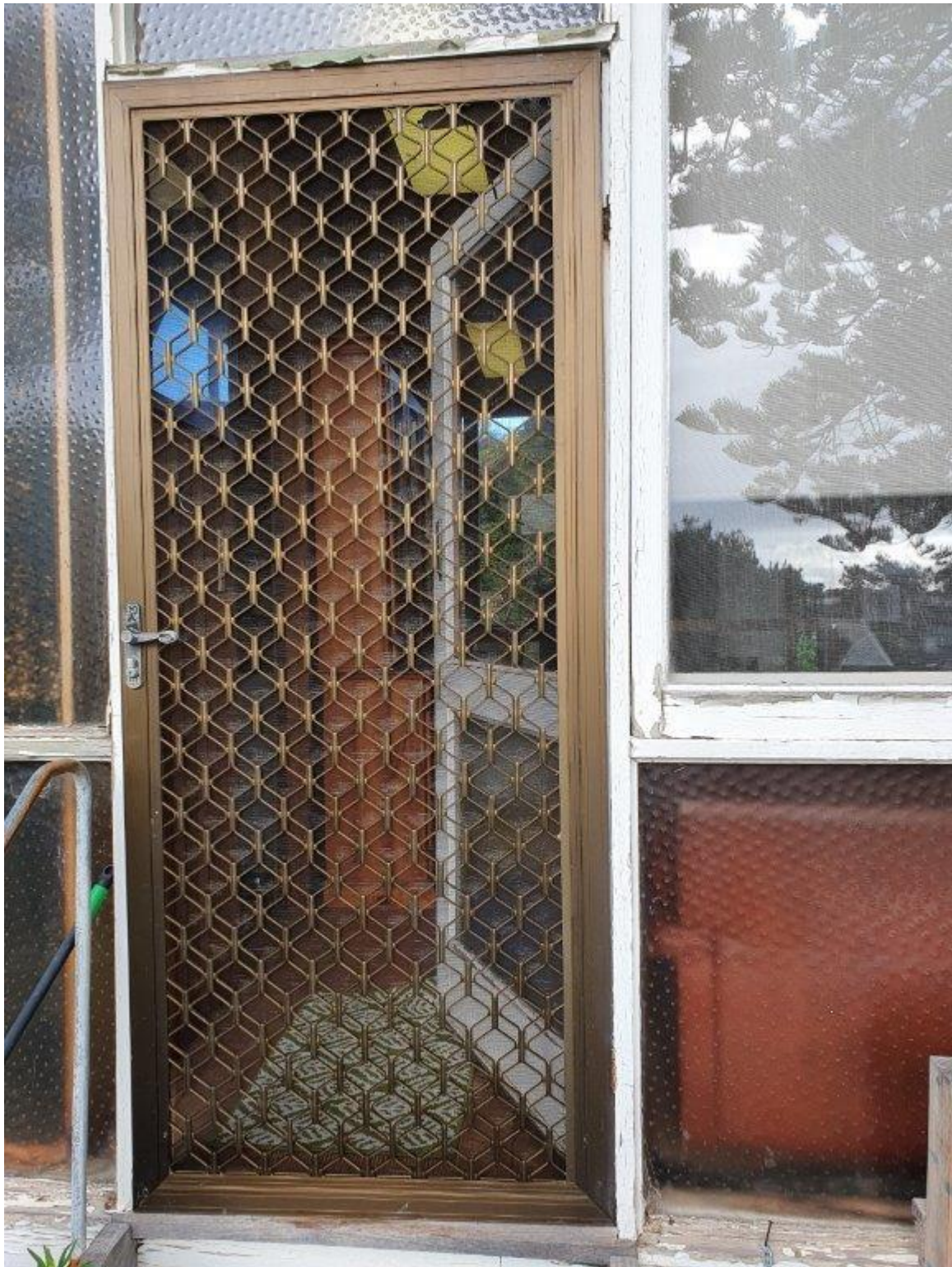
Aframe back door: doorframe misalignment, building movement
