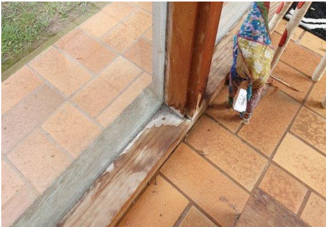
Passageway: water damage
