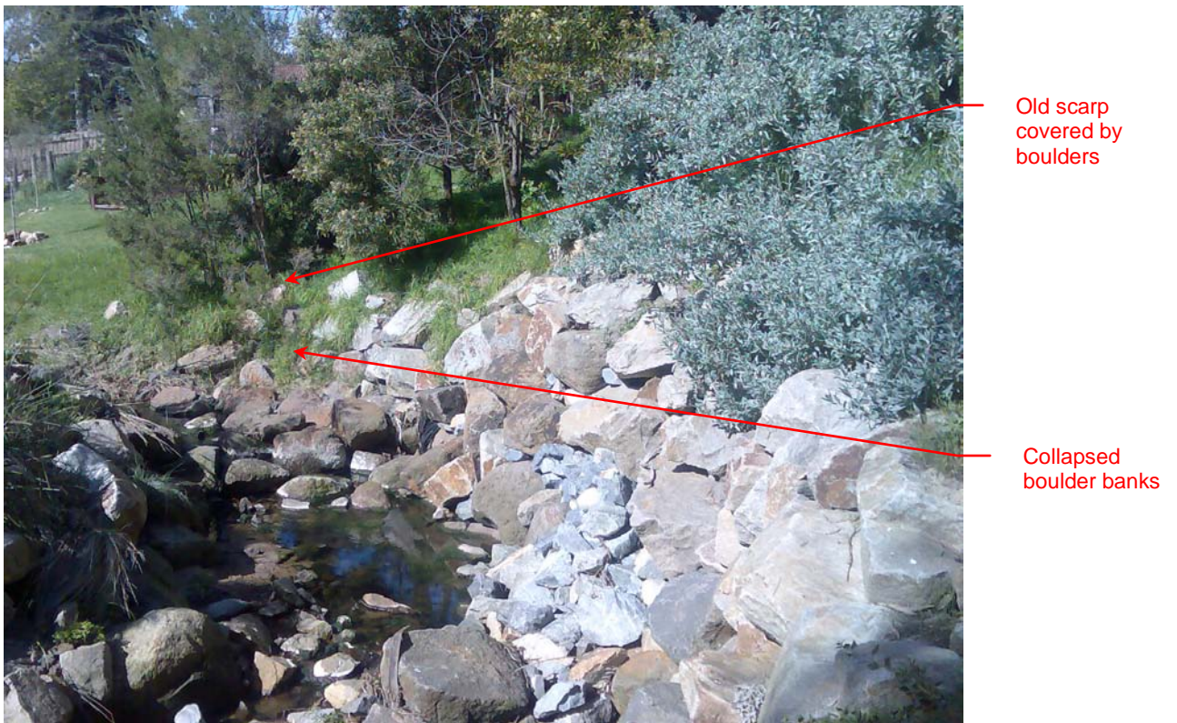
Figure 9-6: Collapsed rock lining behind 11 Shelbourne Court
