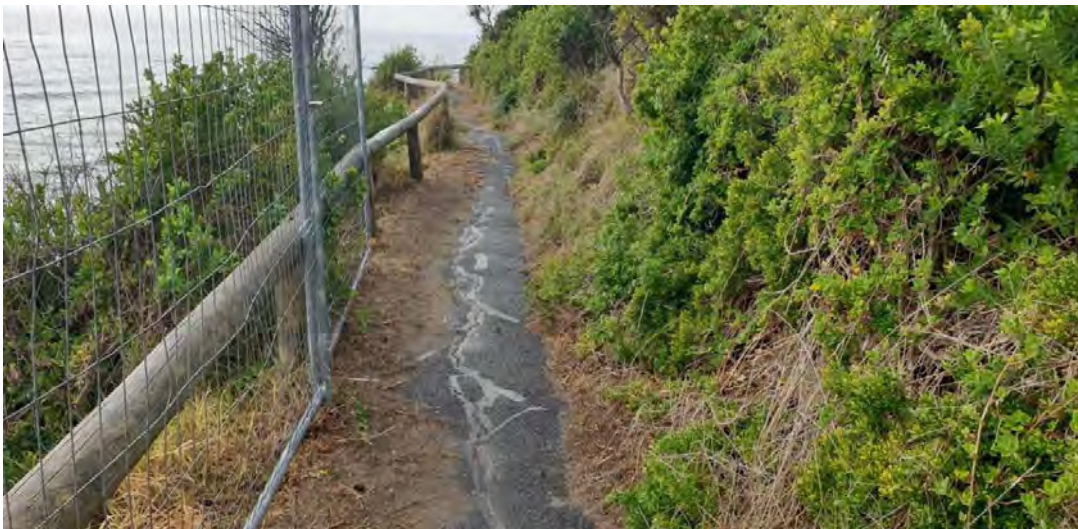
Figure 4-7 – Example of straight cracking (Section 22)
