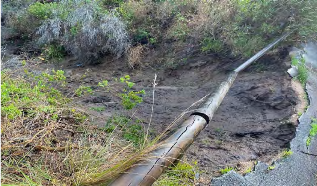
Figure 4-11 - Section 7: Recent Landslide, 2022
