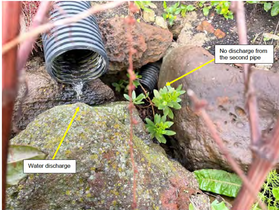
Figure 4-20 – Not all pipes positioned to discharge on the beach had water coming out of them (Section 19).
