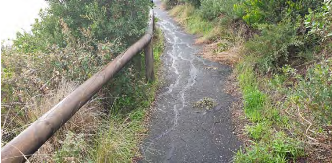
Figure 4-8 – Example of arcuate cracking (Section 16)
