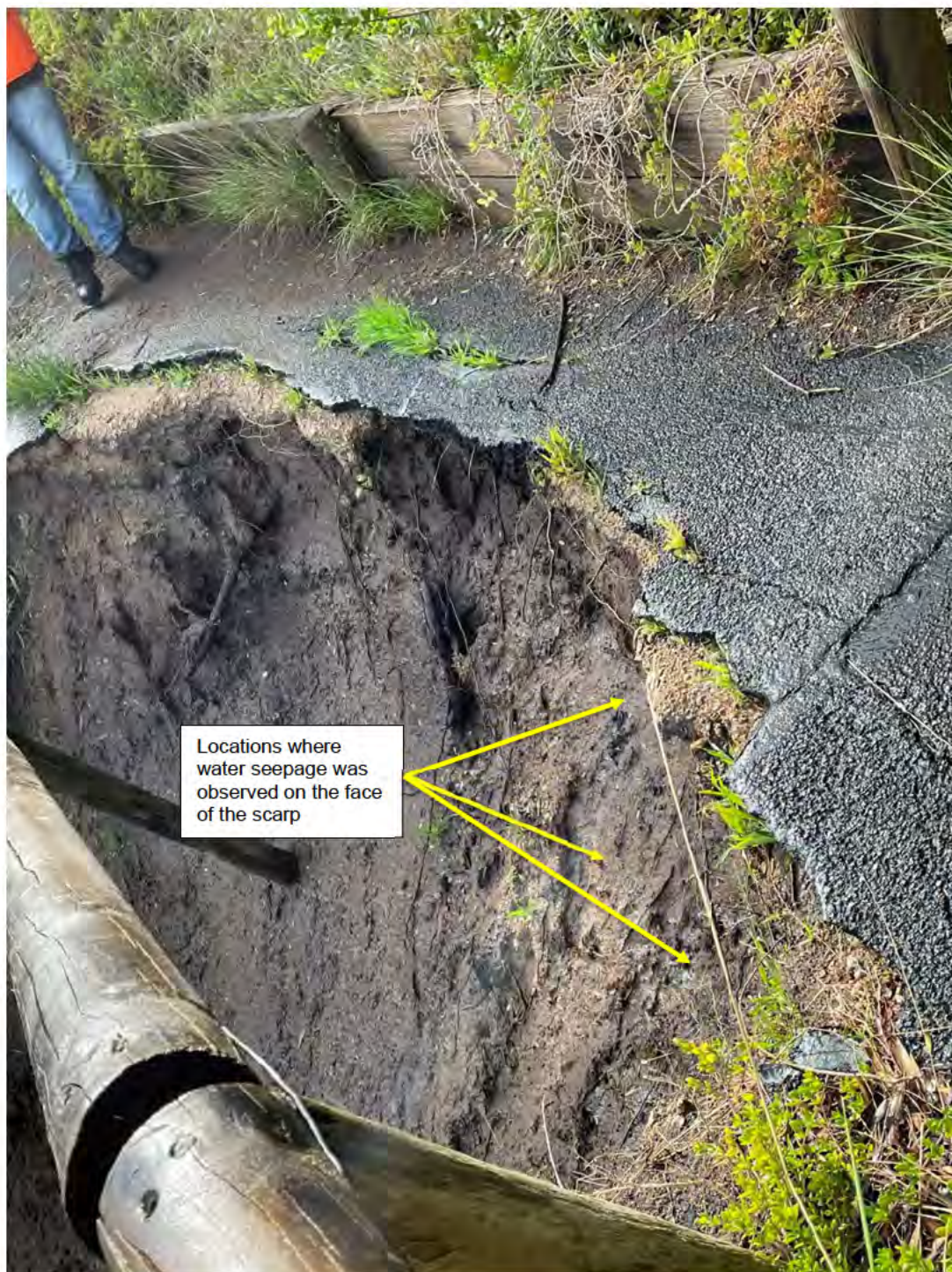
Figure 4-17 – Water seepage observed on the scarp (Section 7).
