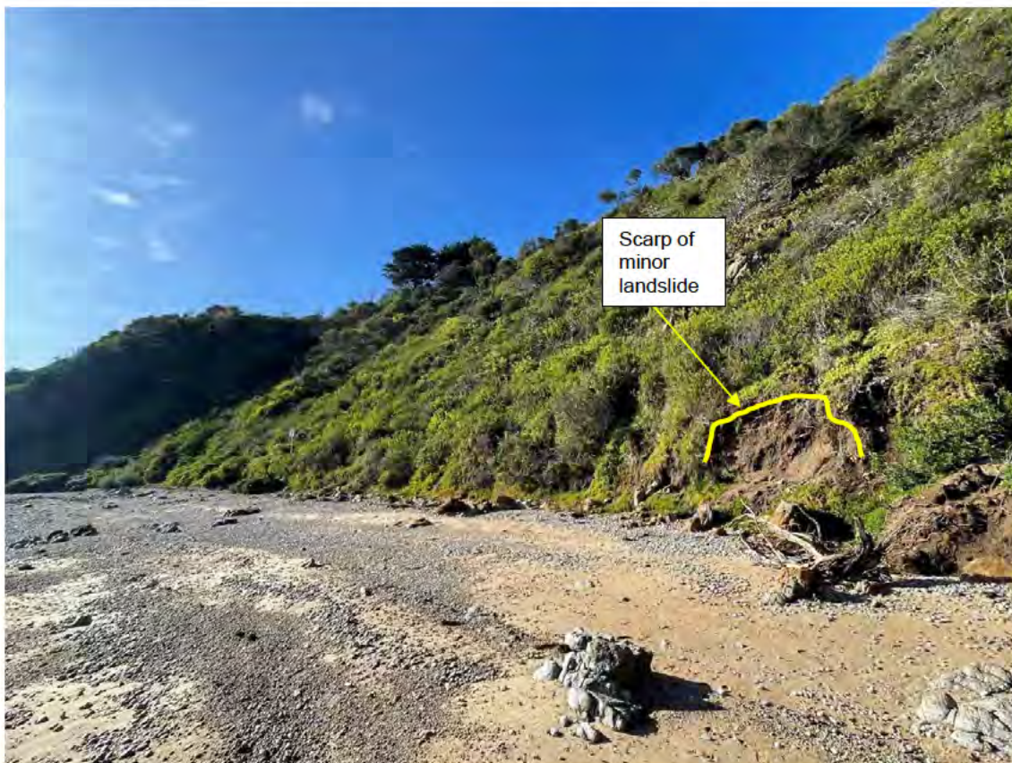
Figure 4-22 – A view of the cliff from the beach
