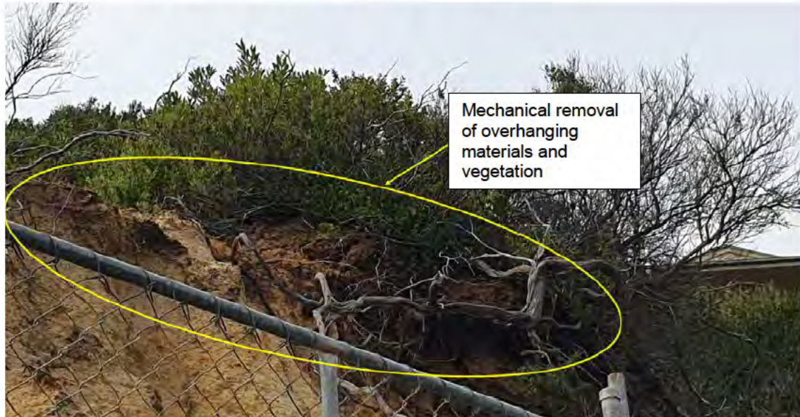
Figure 6-6 – Section 19: zone of overhanging material to be mechanically removed
