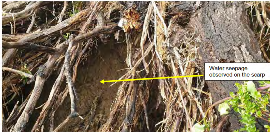
Figure 4-18 – Water seepage observed on the scarp (Section 20).
