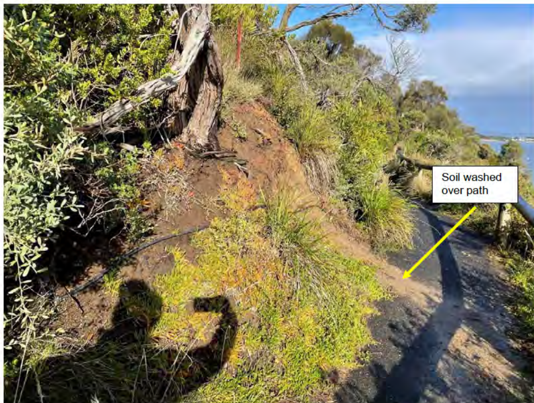
Figure 4-19 – Surface water run off has resulted in material deposited on the path (Section 8).
