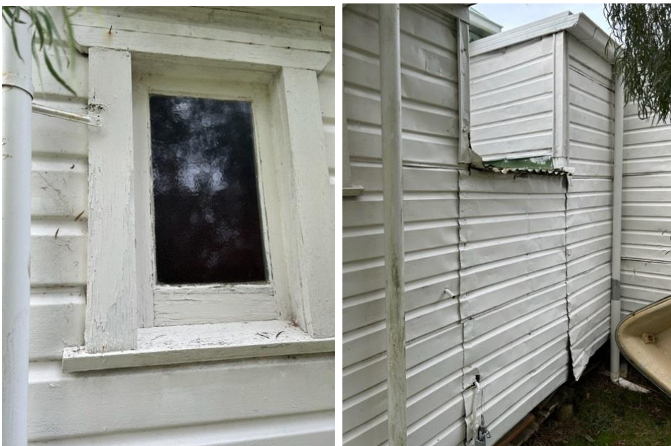
Cladding totally at the end of life. Patched extensively, rusting from both sides.
