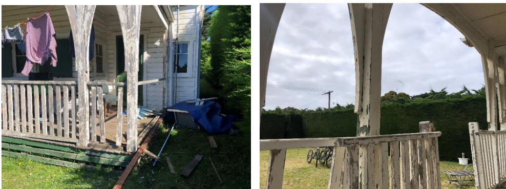
Timbers have been temporarily propped up, but you can see the condition of the timber – it has failed.
