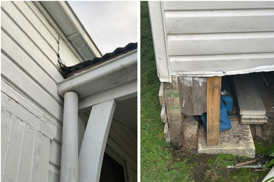
Temporary flashing to cover large rust area, 4 stumps, including latest temporary support with concrete pad sitting on surface. Extensive rust on cladding and bottom section falling off.
