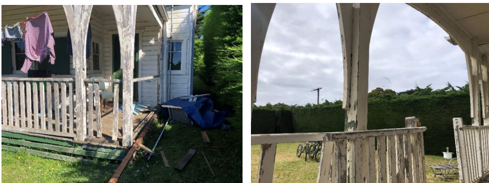
Timbers have been temporarily propped up, but you can see the condition of the timber – it has failed.
