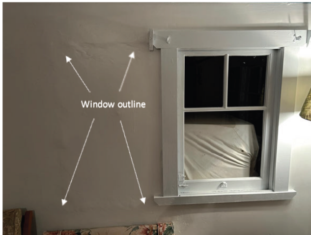
Covered up window between Lounge and Bed 2
