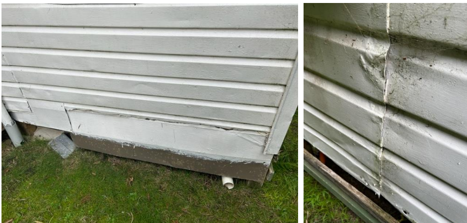
Various patching to exterior cladding to cover rusted out sections.
