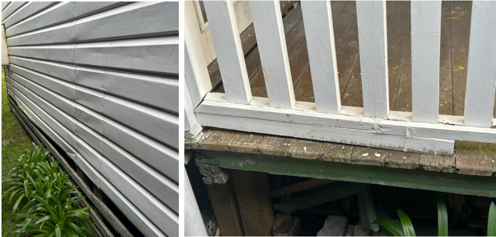
Substructure, stumps, bearers, and beams failed. Temporary concrete blocks to stabilize a 12 – 24 month proposition at best as the reactive clay soil moves up and down depending on seasonal moisture.
