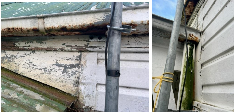
Gutters and drainage dilapidated.
