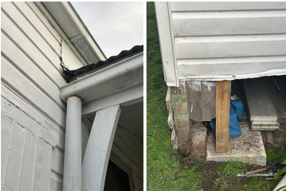
Temporary flashing to cover large rust area, 4 stumps, including latest temporary support with concrete pad sitting on surface. Extensive rust on cladding and bottom section falling off.
