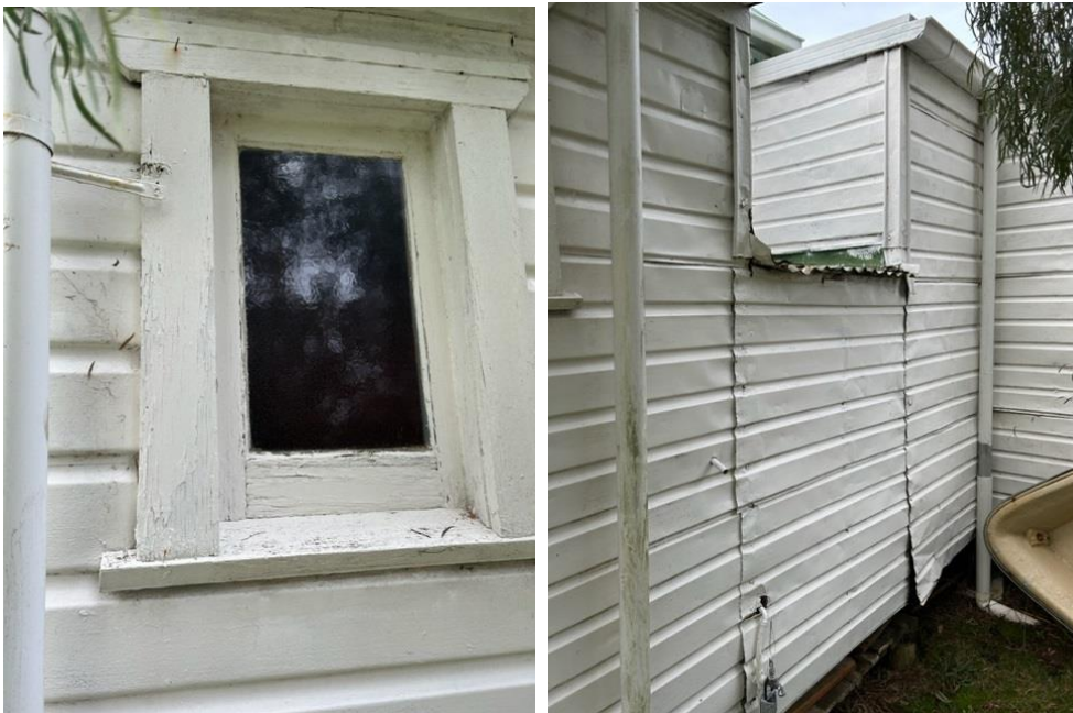
Cladding totally at the end of life. Patched extensively, rusting from both sides.
