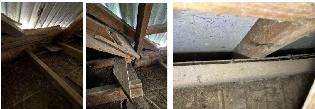
Photos of the veranda centre, photo on right showing external wall with veranda joist connected on the outside of the wall studs and cladding.
