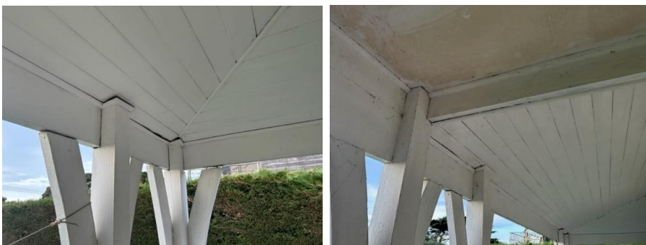
Miss aligned structure supports.
