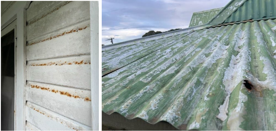
Extensive rust to all cladding. Roof leaks and has extensive holes.
