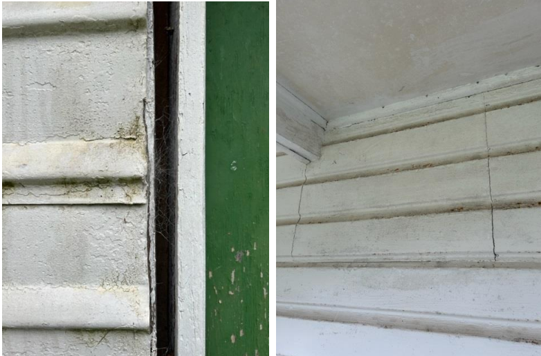
Wide Gaps are throughout the house, vertical cracks in the cladding
