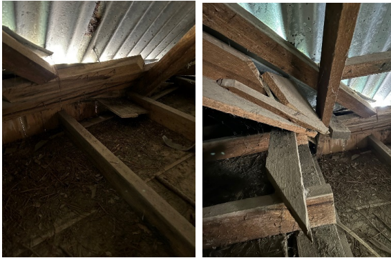
Photos of the veranda centre, photo on right showing external wall with veranda joist connected on the outside of the wall studs and cladding.
