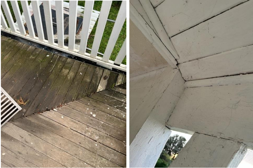
Extensive failure of structure – joints 5mm – 50mm separations. Rotting timbers, total failure.
