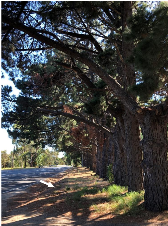
FIGURE 8 RECENTLY FORMED BATTER AT THE BASE OF THE MONTEREY PINES ROW (TREE 101)
