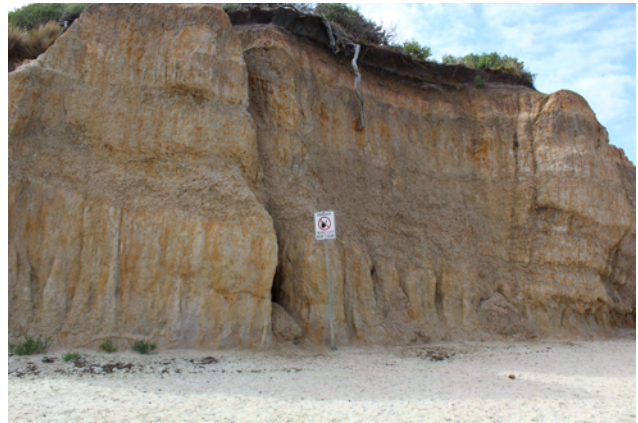
Erosion at Tassell's Beach cliffs
