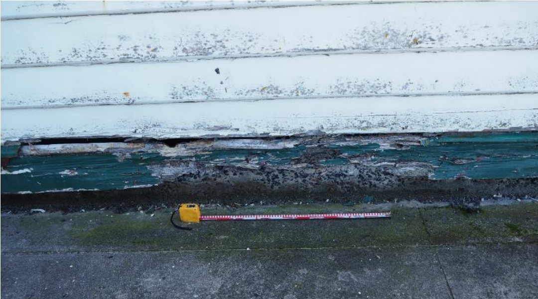
Figure 84: Rotting plinth board on south side of shed.
