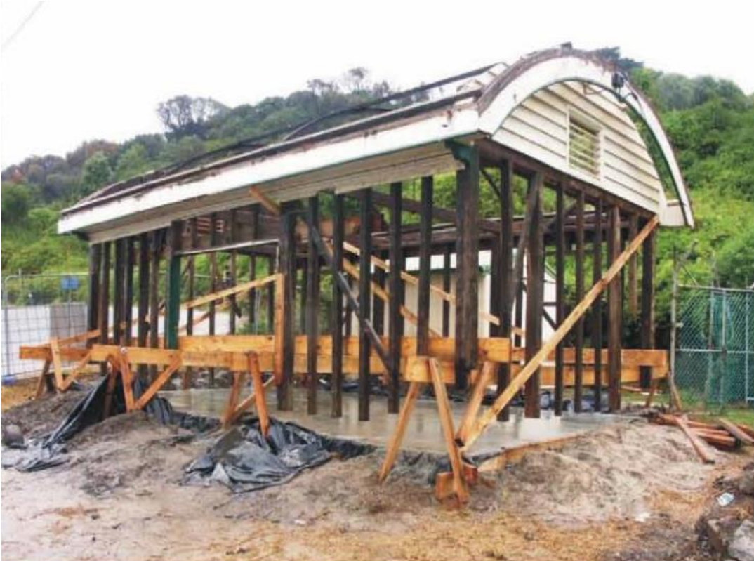
Figure 79: Cargo shed during restoration showing new concrete floor slab and wall studs cut at base for scarfing
