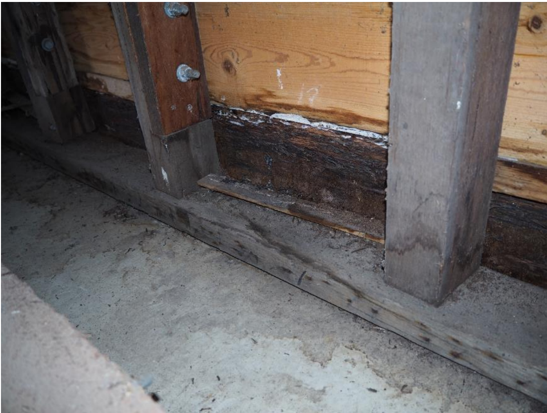
Figure 82: Damaged timber on inside of plinths
