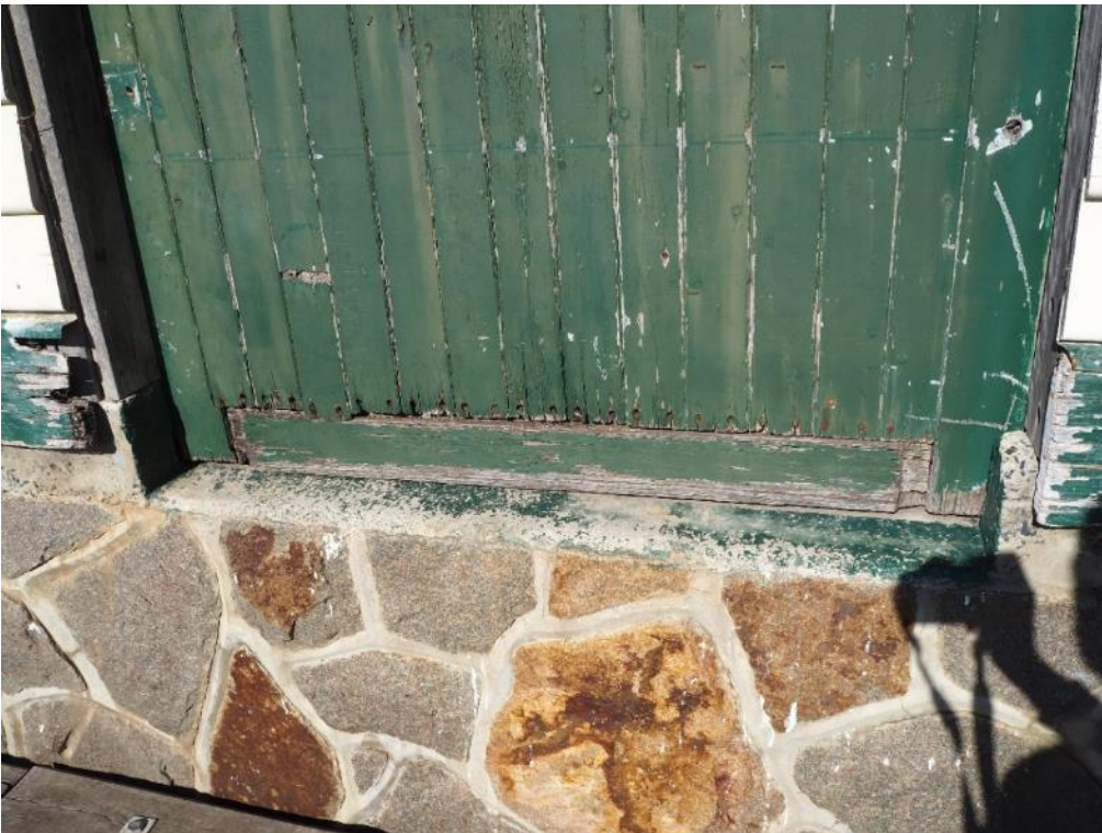
Figure 85: Rot and detached timbers at base of north door and plinth
