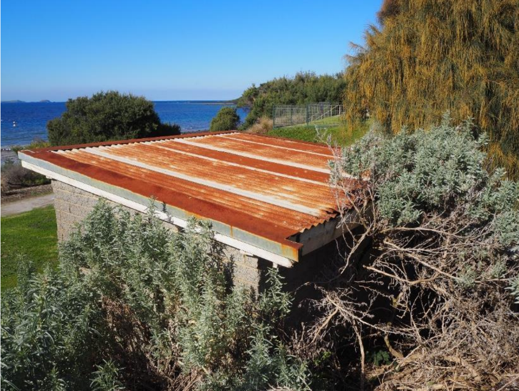
Figure 87: Winch shed roof showing rusted lower end of iron
