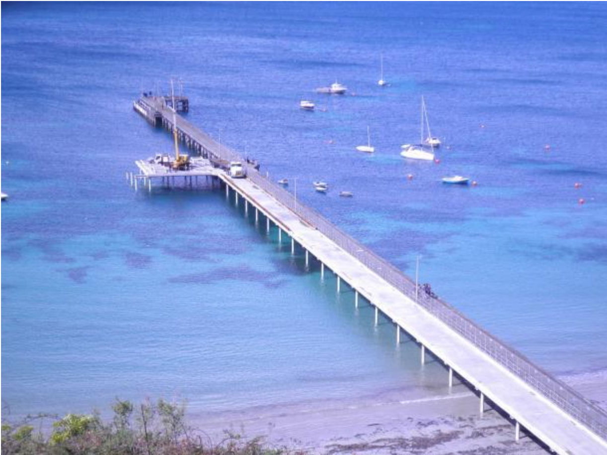
Figure 36: Flinders Pier during construction of new section 2011 to serve commercial vessels including the pilot boat
