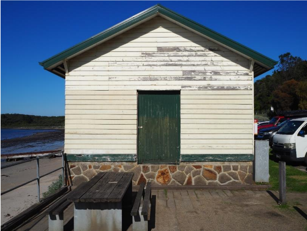
Figure 55: North elevation showing deteriorating paintwork (G. vines 2023)
