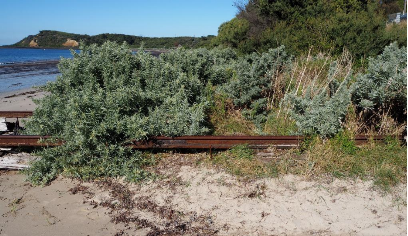
Figure 60: Buried section of slipway with supporting timbers collapsed (G. Vines 30/5/23)
