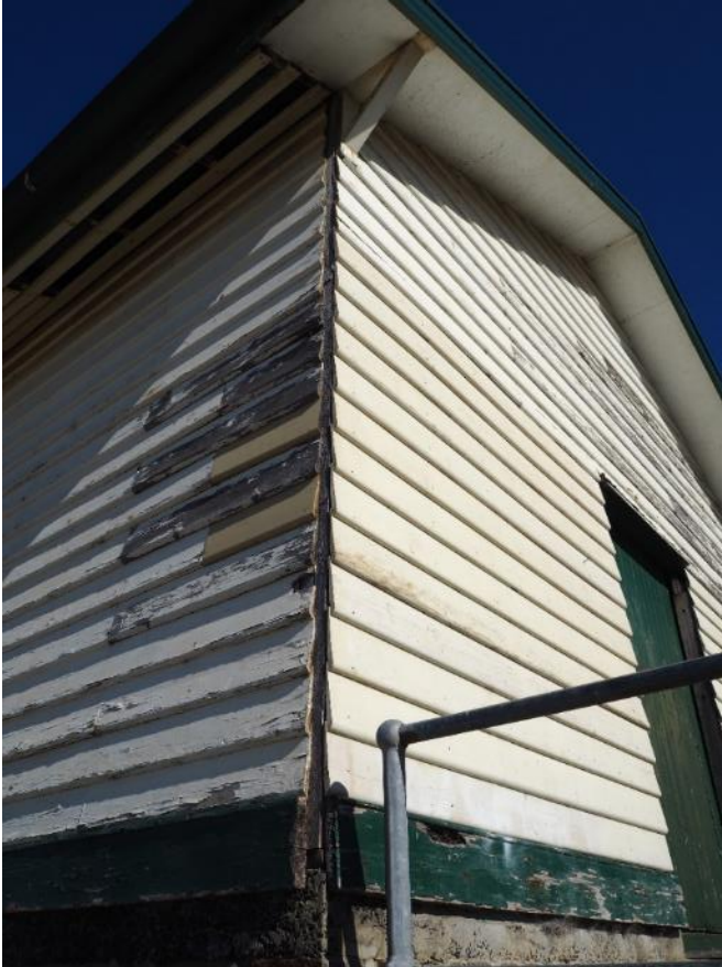
Figure 86: Deteriorating plinth boards, corner and flaking paint on weatherboards
