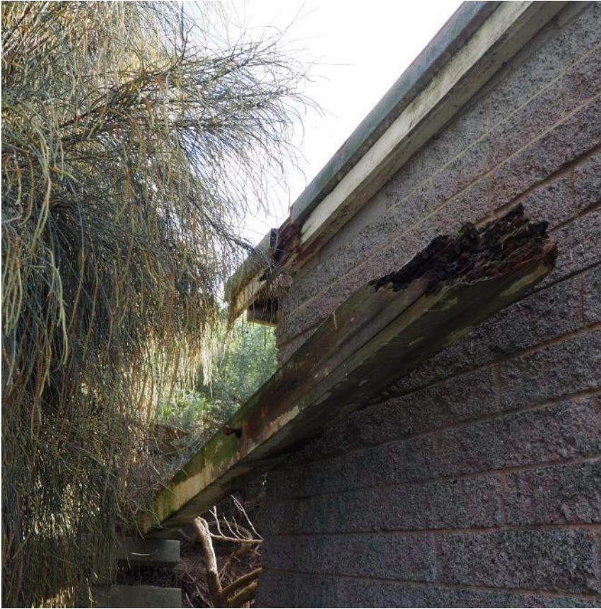
Figure 89: Rotted remnant of electricity pole on south side
