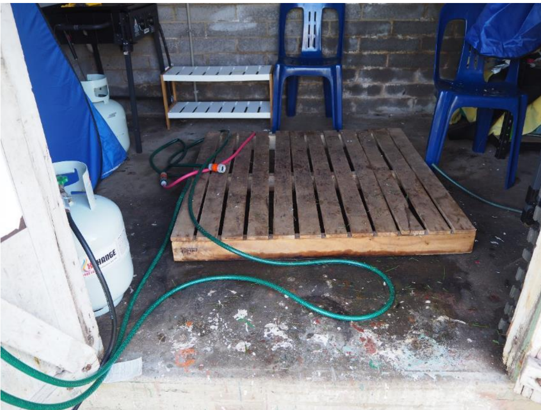
Figure 90: Interior concrete floor showing damp from shower splash
