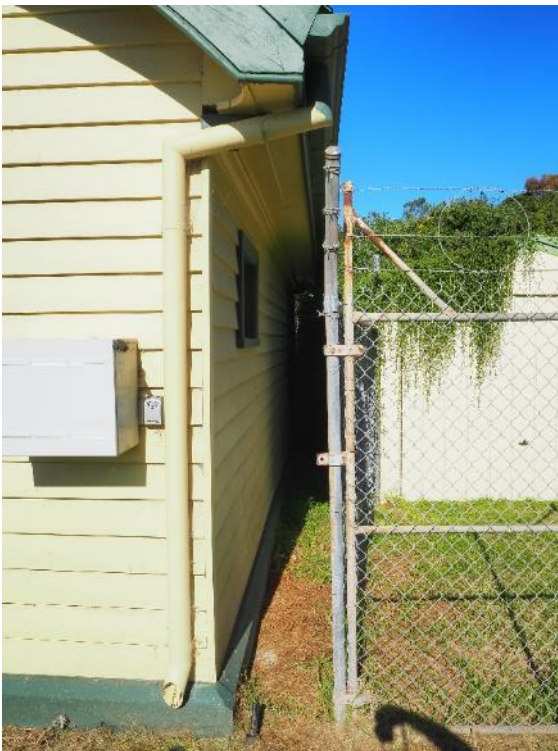
Figure 80: Vegetation encroachment and insufficient access at rear of Cargo shed
