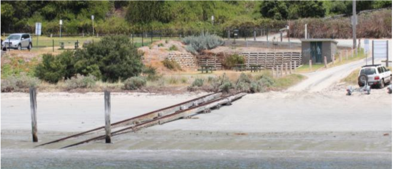
Figure 58: Slipway from the pier, note winch shed, and recent concrete crib retaining wall (G. Vines 2013)
