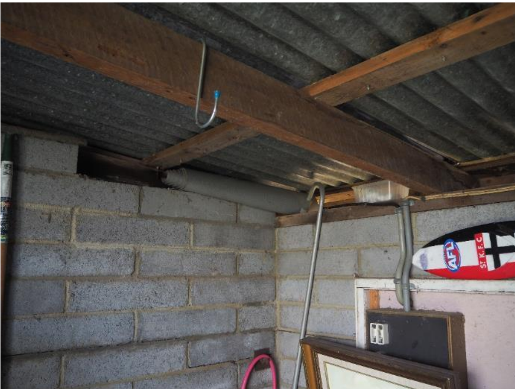
Figure 88: Shed interior showing damp coming through mortar course
