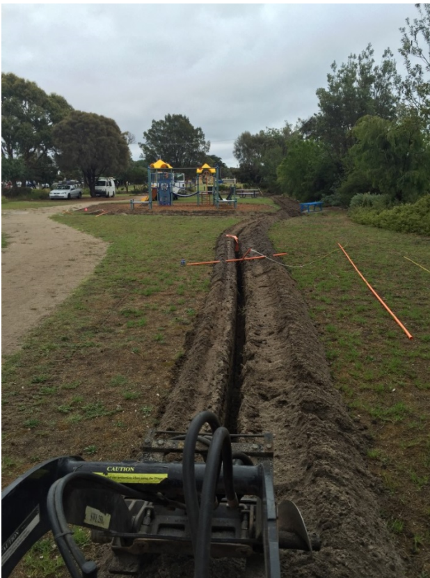
Image: Lighting conduit installation works associated with the Western Connecting Path and Laneway (adjoining the Rosebud Bowls Club)
